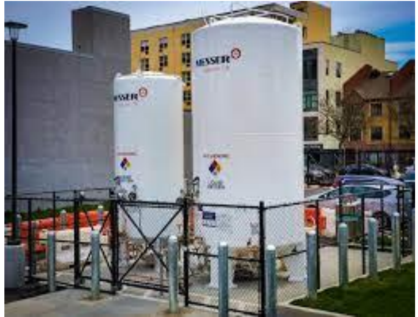
Liquid Oxygen supply system
