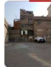
Bad condition(Old house)
