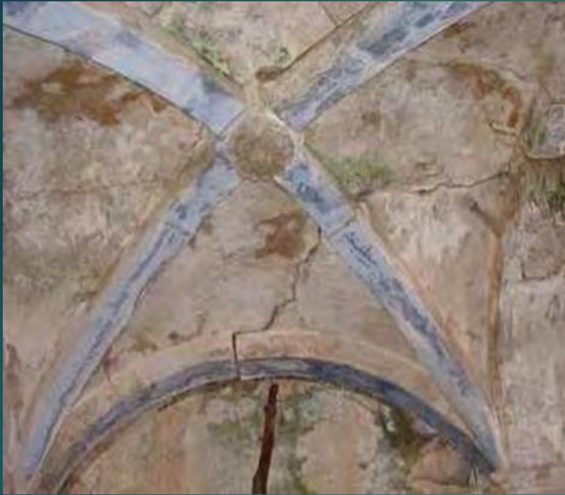
Figure.5 : Cracks in a masonry vault
