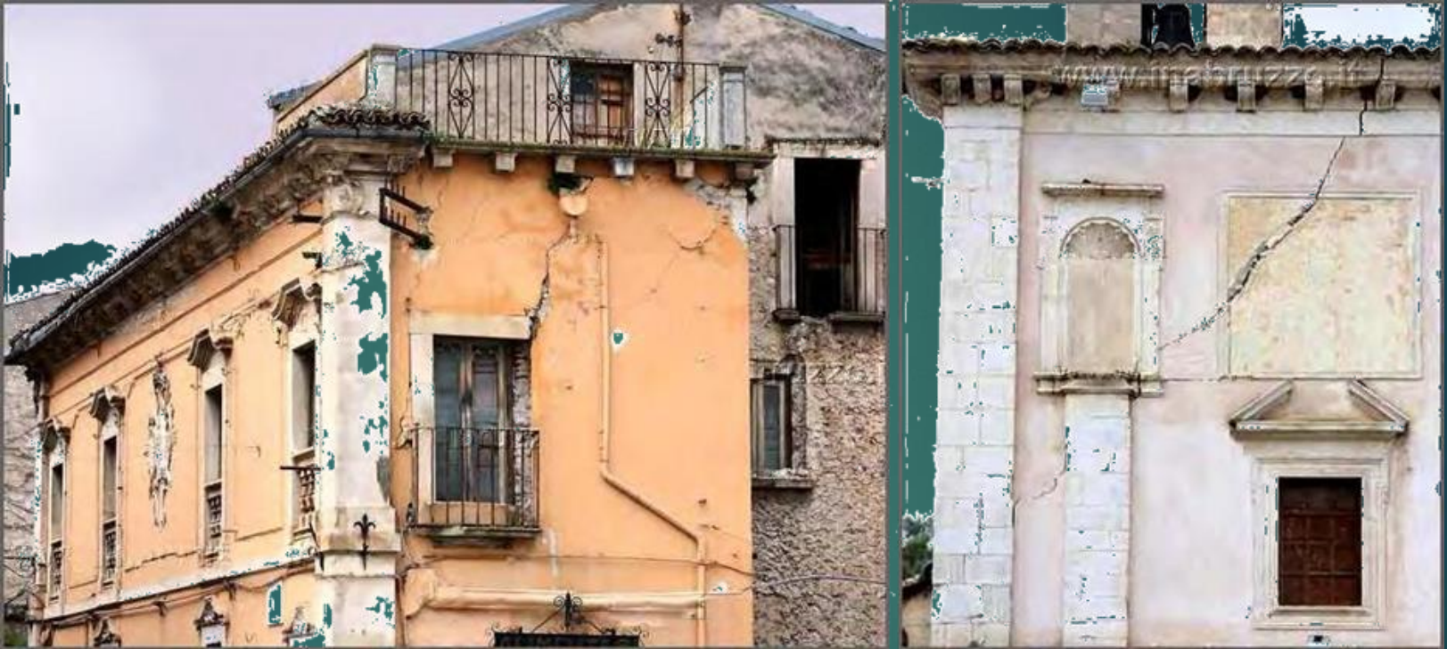
Figure.4 : Damage in walls due to earthquakes
