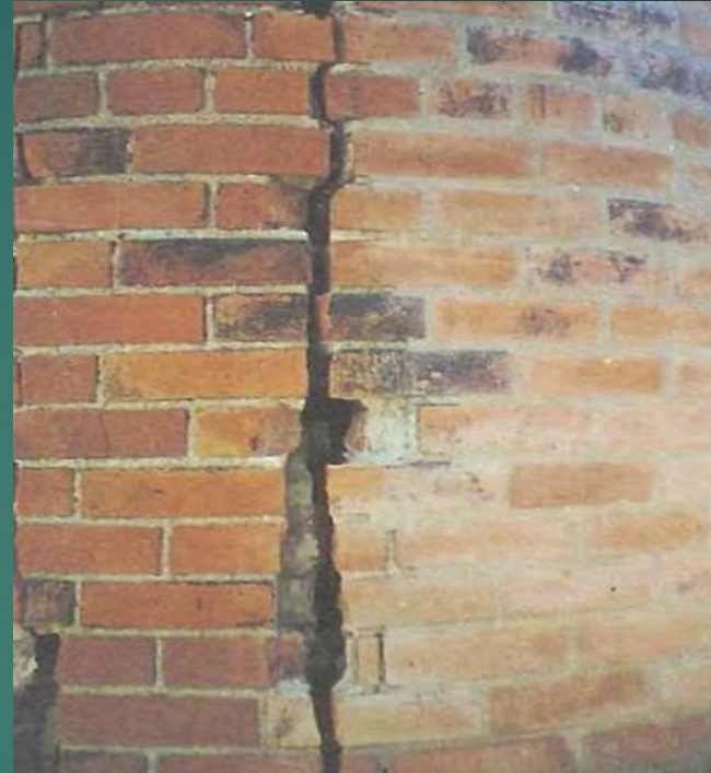
Figure.6: vertical cracking in masonry chimney
