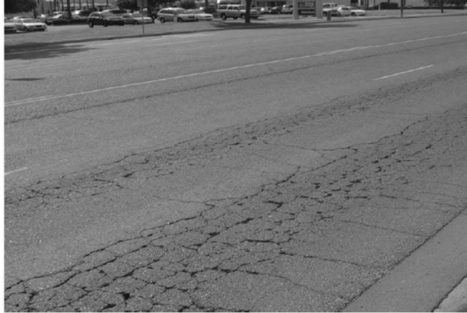
FIGURE 1.17 Fatigue failure of asphalt pavement due to repeated traffic loading.
